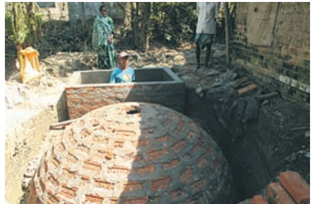
Bio gas at Haldia
