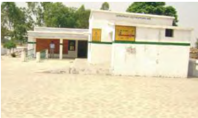
Boundary wall and pavement of the school ground completed at Dadpur School
