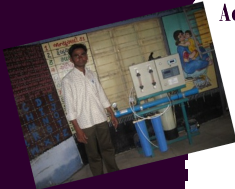
RO Plant at Gadechi School
