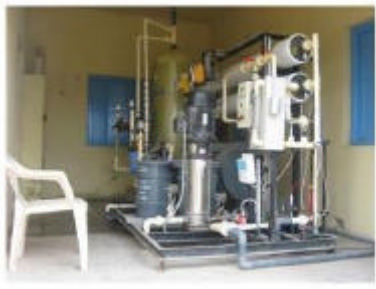
Reverse Osmosis Plant (RO plant)
